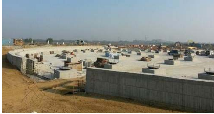
Figure 8: General view of the installed sliding pendulum
