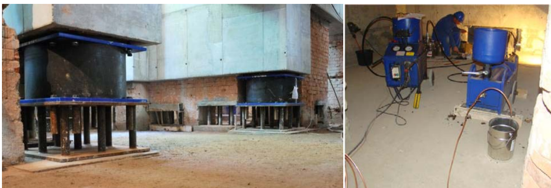
Figure 7: HDRB before grouting the lower frame (left) and during the load transfer (right)
