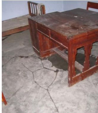
Figure 7. Ground fissures caused by liquefaction ejection at Tian'e village, Lichun town
