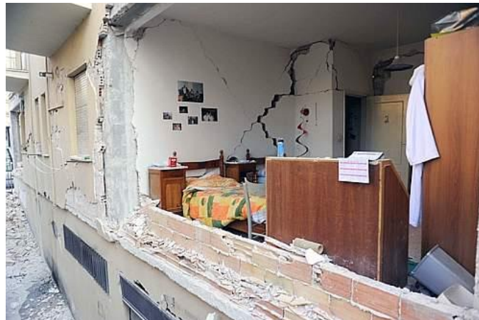
Figure 3. Damage of apartment building in l'Aquila, Italy after April 6, 2009 earthquake
